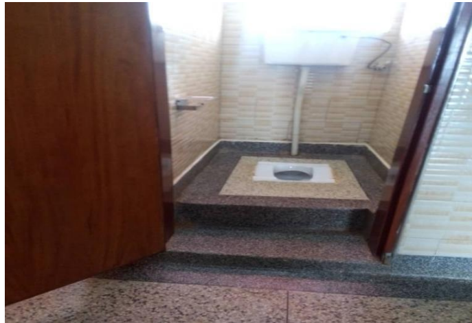
Figure 2. Water Flush Toilet at Campus B
