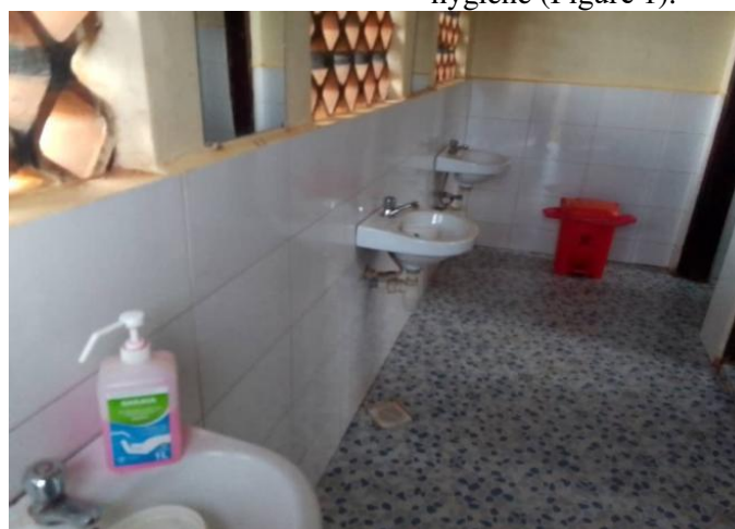
Figure 1. Indoor Hand-washing Facility with Limited Natural Lighting, Campus B
