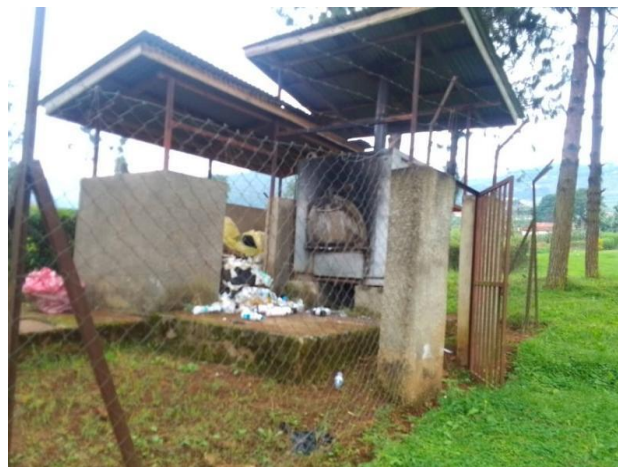
Figure 8. Dysfunctional Incinerator, Campus B
