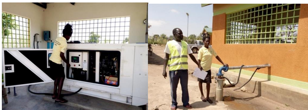
Plate 4. 1: Chlorination System at Imvepi 1
