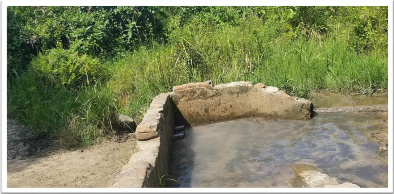
Bung Amon Protected spring flooded with drainage line blocked and no diversion line for surface run off for water.
