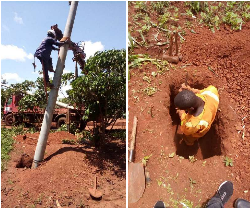
Figure 4. 8: Digging of the hole using a crowbar and hammers (right) and erection of electricity poles (Left) by workers on the worksites
