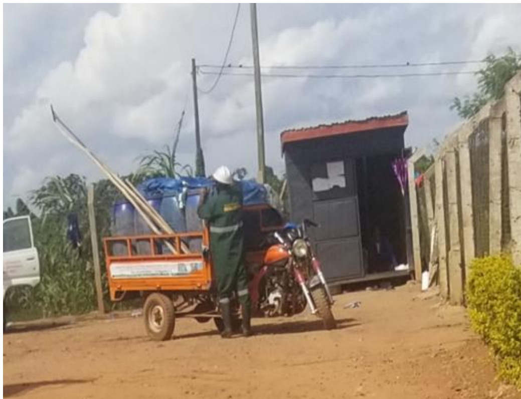
Figure 26 Showing a gulper pipe and drums on the tricycle.
