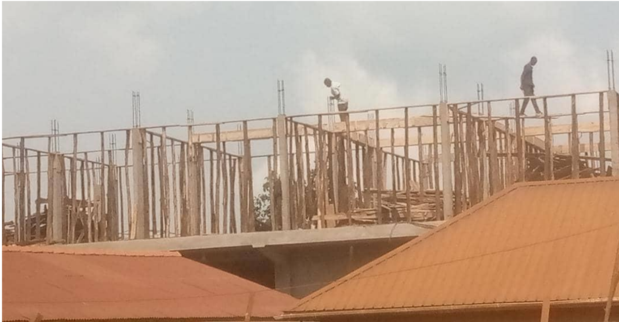
Figure 4. 4: Workers walking on top of pillars on a building construction site in Kira Municipality without scaffoldings and PPE, exposing them to occupational falls
