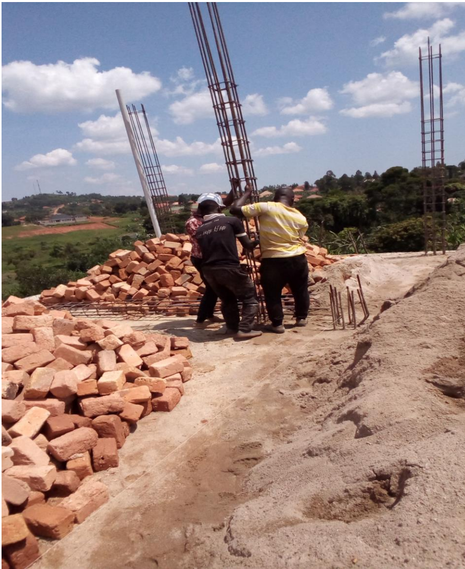
Figure 4. 5: Workers erecting iron bars at a building construction site in Kira Municipality without PPE like gloves and safety shoes making them exposed to skin cuts and pierces
